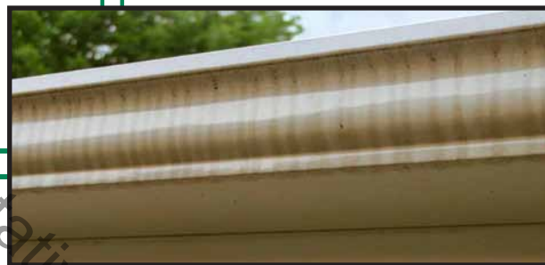
Tiger Striping on Gutters
